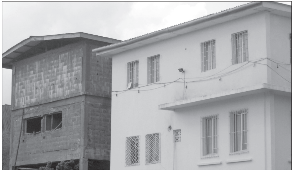
Figure 6: Liberian Ministry of Lands, Mines, and Energy Building and Secured Annex under Construction for Housing Liberia's Rough Diamond Exporting and Importing Authority
