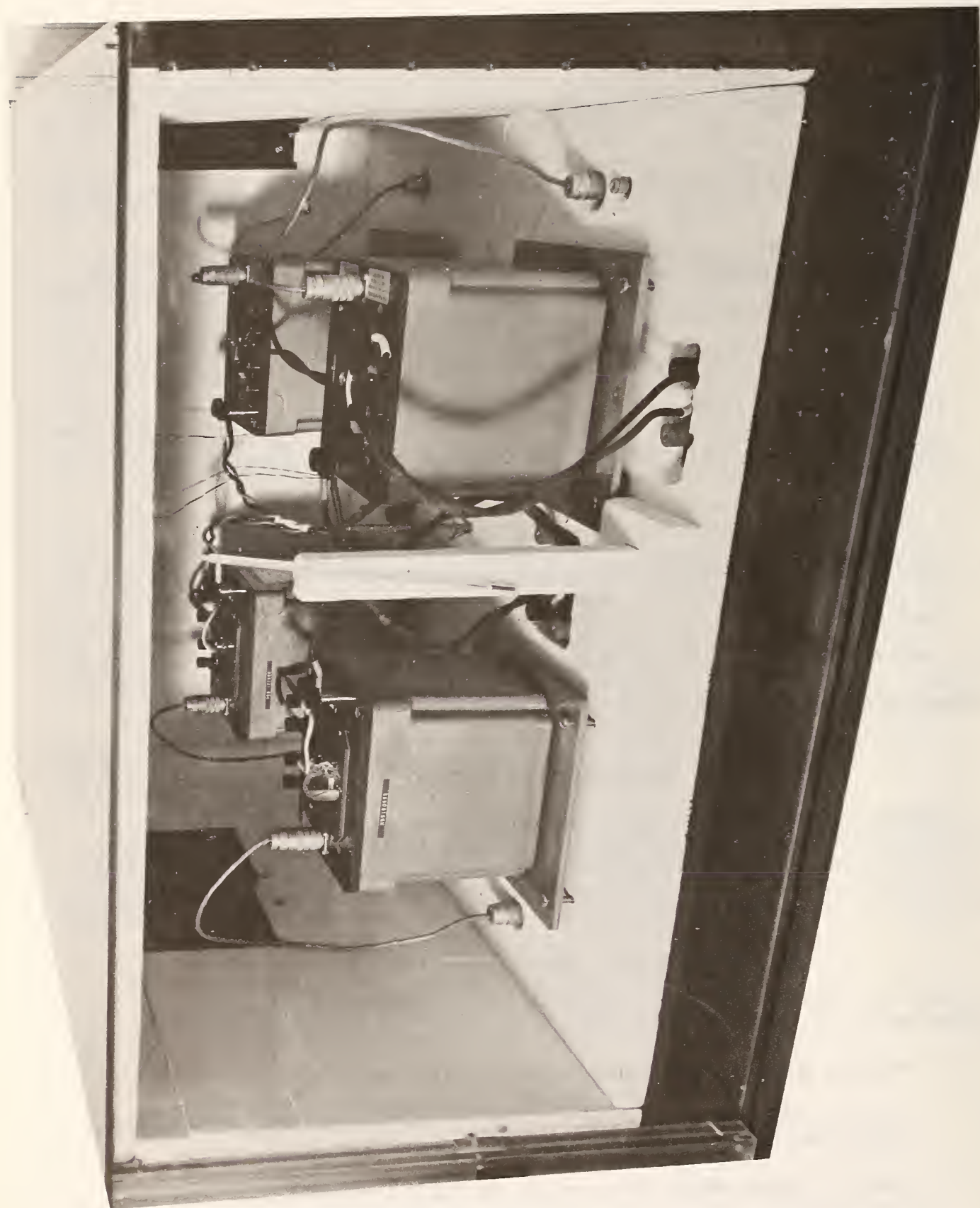
Figure 5-1. View of the four rotating watt-hour meters inside the thermally controlled enclosure. These meters comprise the NBS reference bank.
