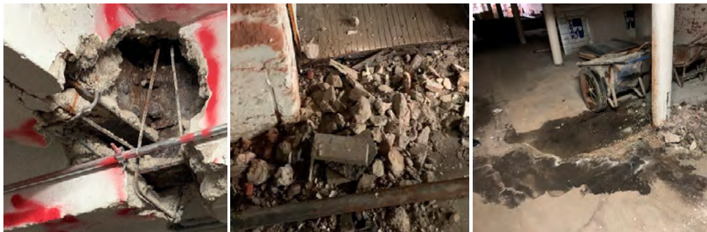
Above left to right: crumbled cement from ceiling joist, pile of crumbled cement, and moisture in area of crumbled cement
