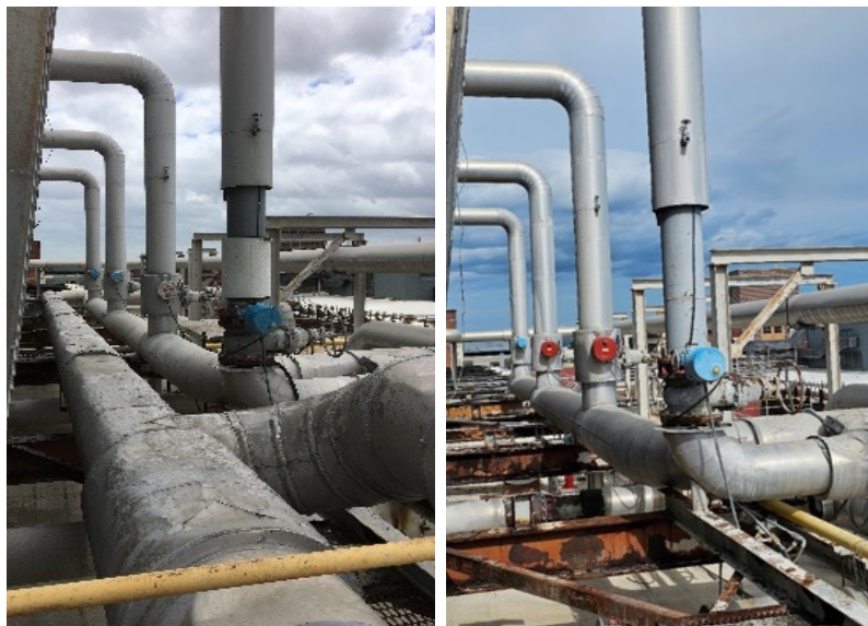
Before and after photos with insulated piping in place and with insulated piping removed
