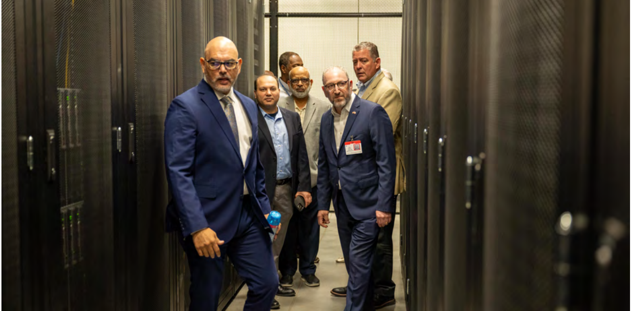
GPO's state-of-the-art data center at the Iron Mountain facility in Virginia boasts 55 physical servers and 800 virtual servers. This three-year project completes a major upgrade initiative for the digital side of GPO operations.
