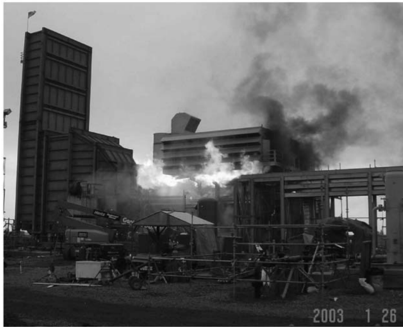
Figure 4. Previous explosion during a natural gas blow on January 26, 2003, at a Calpine natural gas power plant in Fairfield, California. The explosion was heard 10 miles away.
