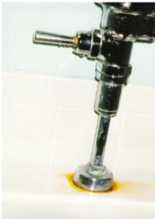
Figure II.8: Leaking and Stained Urinal in Public Rest Room at Shenandoah National Park
