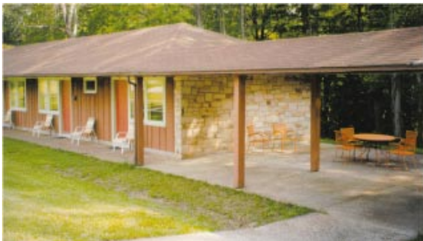
Figure II.7: Needed Exterior Repairs at Mammoth Cave Lodge
