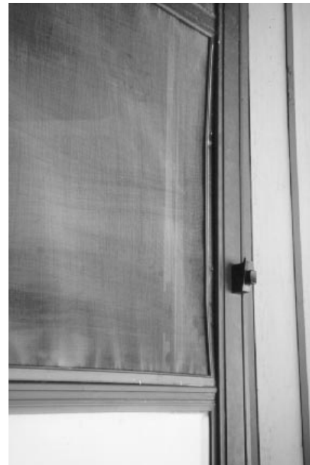
Broken handle and screen on back door
