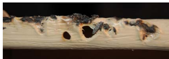
Image of vinyl siding (from bottom) after firebrand exposure at 7 m/s
