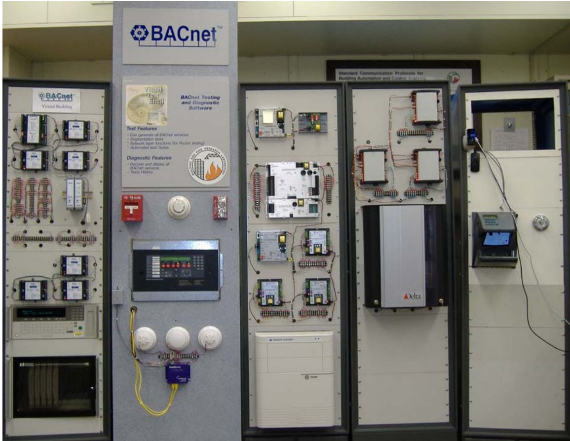
Figure 2. VCBT controller hardware, data acquisition system, fire-related devices including fire-panel, and biometric devices. Workstations for the VCBT controllers are not shown.
