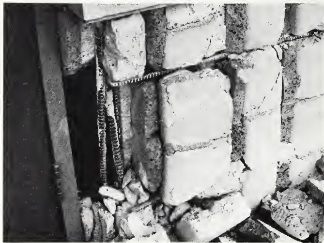
Figure 6 Studies of proper perimeter bar splices in masonry walls should be made.
