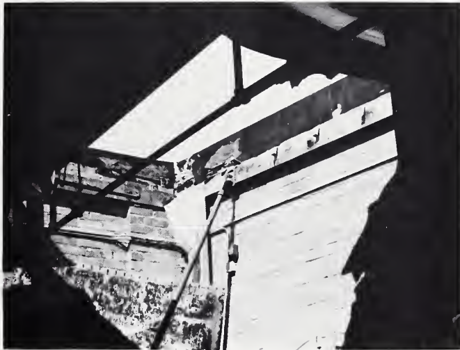
Figure 8 The influence of the corners of masonry walls on the performance of horizontal diaphragms should be examined.
