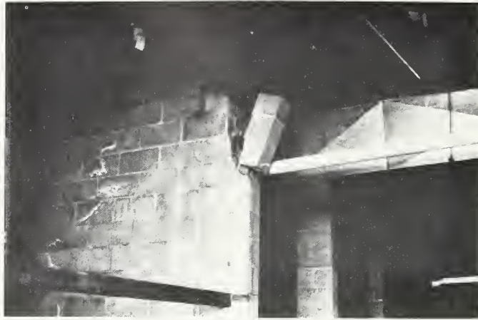
Figure 1 If the vertical trim bars were bent horizontally under beam or if a horizontal hairpin bar were placed around the bolts this damage may be alleviated.
