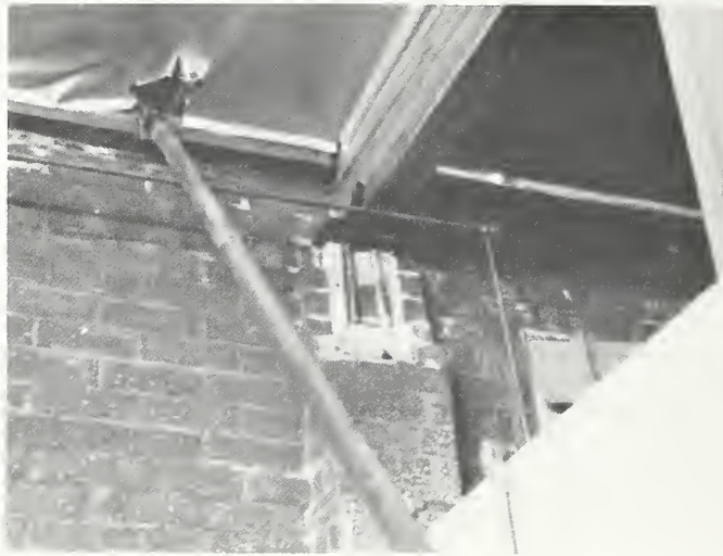
Figure 2 Horizontal ties around the bolts may alleviate this damage and increase their strength.
