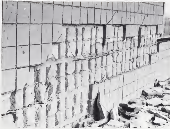
Figure 7 Investigations are needed to improve bonding the face shells of concrete block to the grout core. Note the horizontal pour joint in the grout cores.
