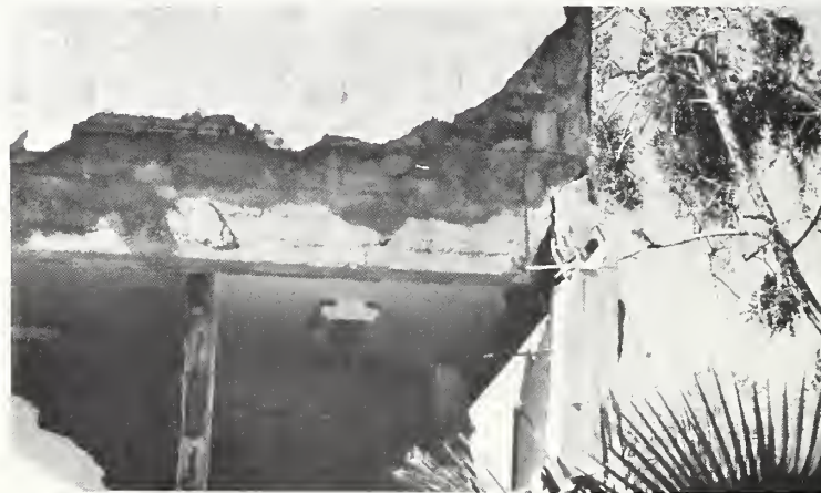
Fig. 18 Detail of Sylmar building showing failure at corner column.
