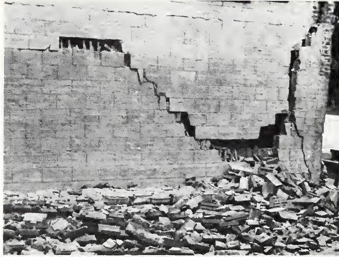
Figure 5 Masonry veneer was shaken from this concrete block wall.
