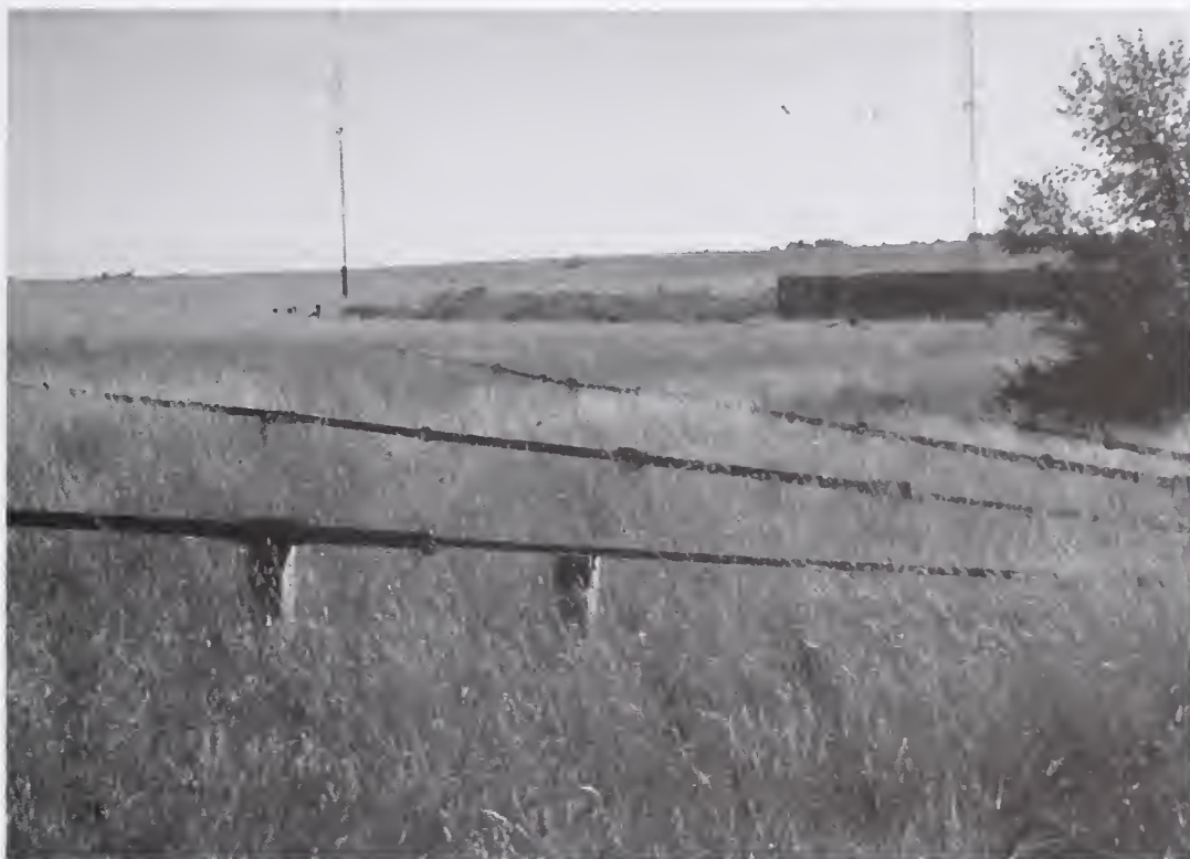
Figure 1.13. Transmitter to antenna transmission lines at WWV.
