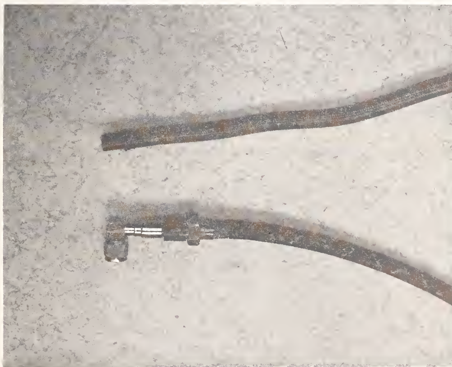
Figure 2. Shielded jumper cable connector assembly and stripped back convoluted shield.
