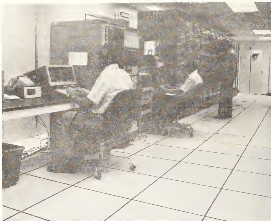
Figure 3. Data acquisition facility main screen room hardware.
