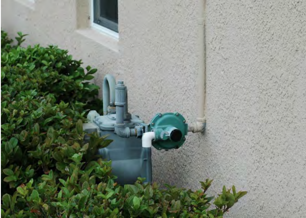
Figure 10 – Gas meter on the outside of a problem drywall home.
