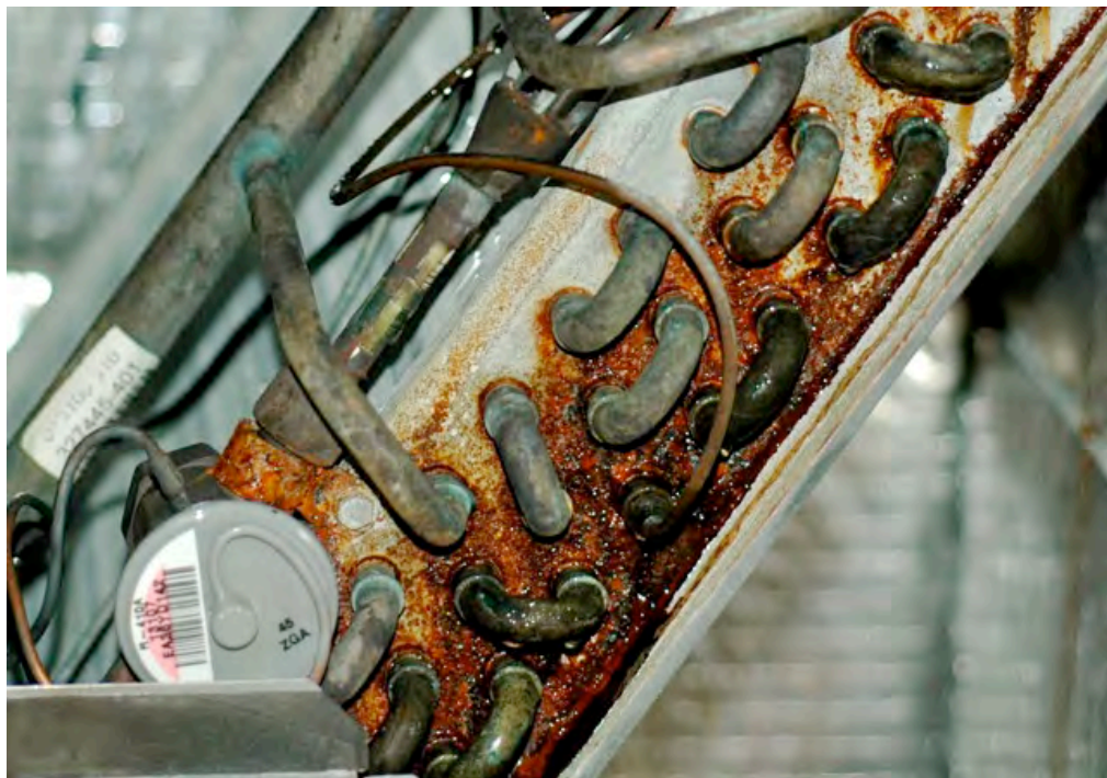
Figure 14 – HVAC unit in the attic of a home with problem drywall.
