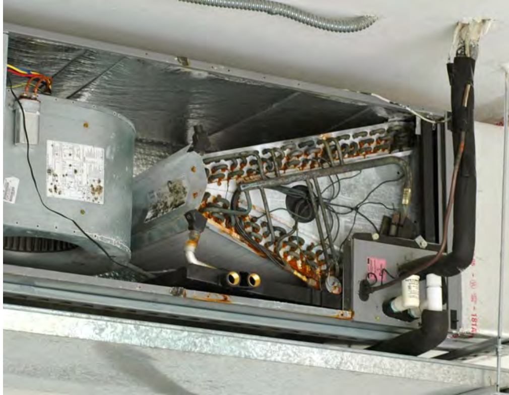
Figure 13 – HVAC unit in the garage of a problem drywall home.
