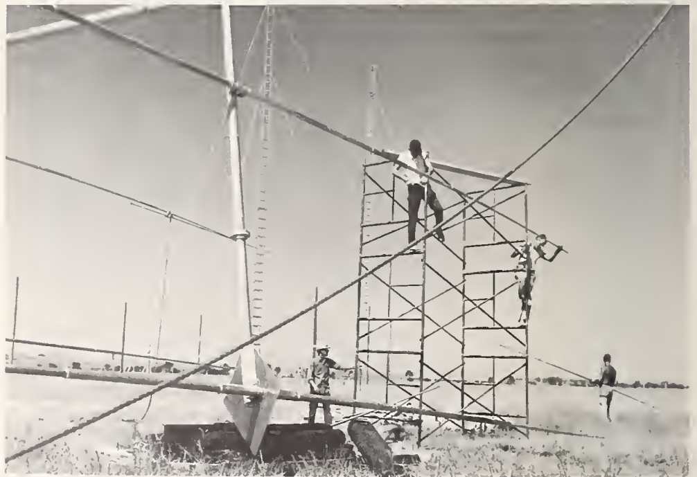
Erection of an antenna at the NBS Erie (Colo.) field site for radar studies of ionospheric irregularities. (See p. 159.)
