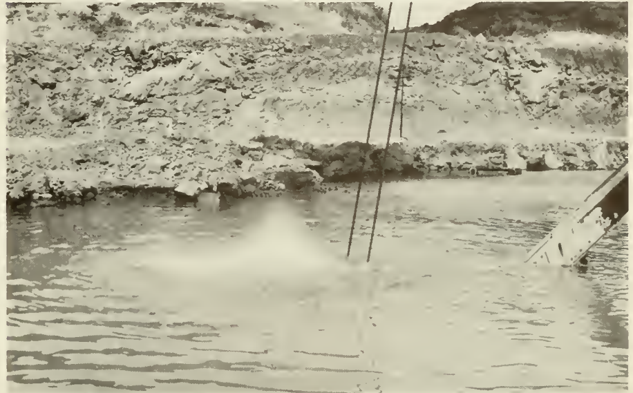
The blast, set off electrically with the rock submerged 8 to 10 feet, cause little surface turbulence. The water reduces the sound of the blast and reduces the "fly" of fragments. The charge for this shot was four sticks of 1¼ by 12-inch 60 percent dynamite. These pictures, taken by a Panama Canal official photographer, were among several used in a recent issue of Engineering News-Record.
