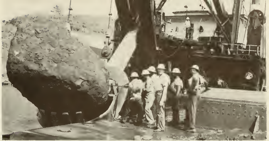
Underwater excavation in widening of the narrowest parts of the Panama Canal from 300 to 500 feet often means encountering big rocks not shattered by banks blasting. Above, in the 13½ cubic yard bucket of a dredge, is a big one weighing between 20 and 30 tons. It is being drilled to take the dynamite charge which will fragment it.
